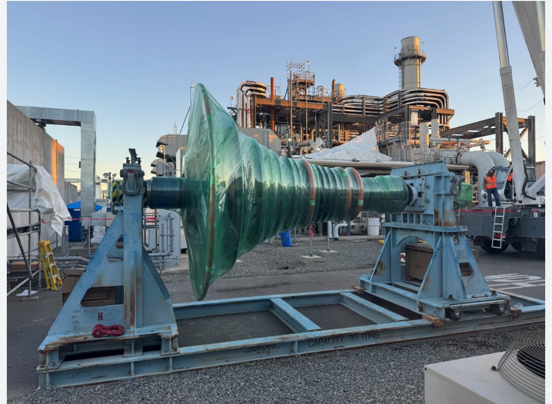
Steam Turbine Rotor
