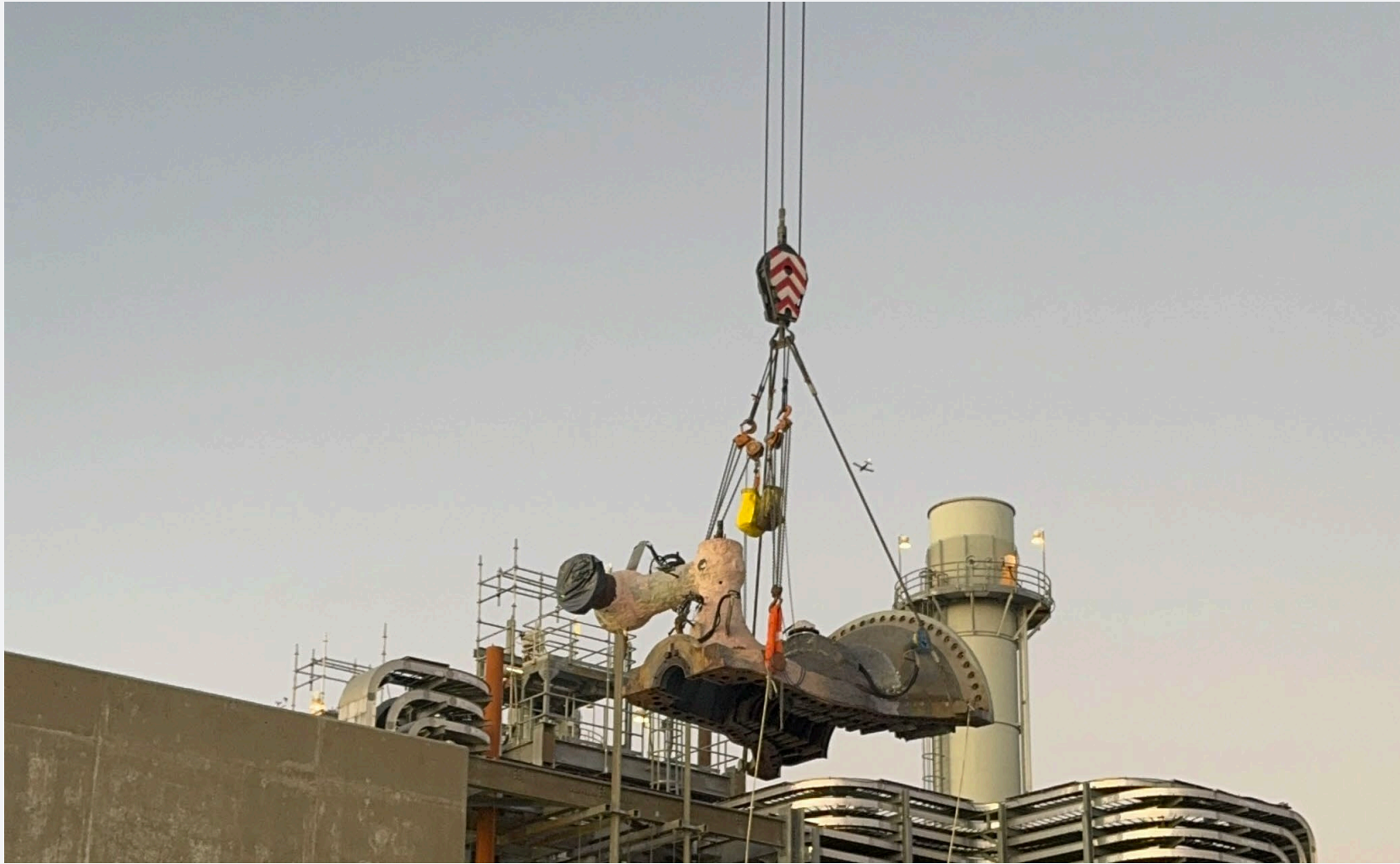
Steam Turbine Top-Case ~85klbs
