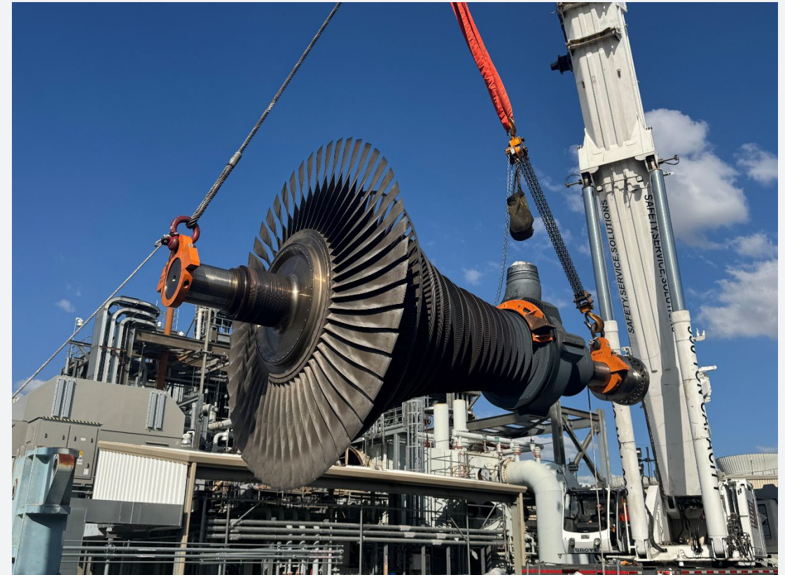
Steam Turbine Rotor ~60klbs
